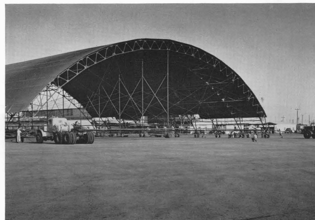
To make room for construction of the new terminal building at Dhahran International Airport, a hangar was "put on wheels" and towed by truck to a different location a quarter-mile away.
